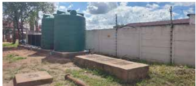
Recycled Water storage for re-purposing
